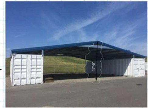
CARGO CONTAINERS WITH ENGINEERED STEEL ROOF CARGO CONTAINERS ATTACHED TO CONTINUOUS CONCRETE FOUNDATION
